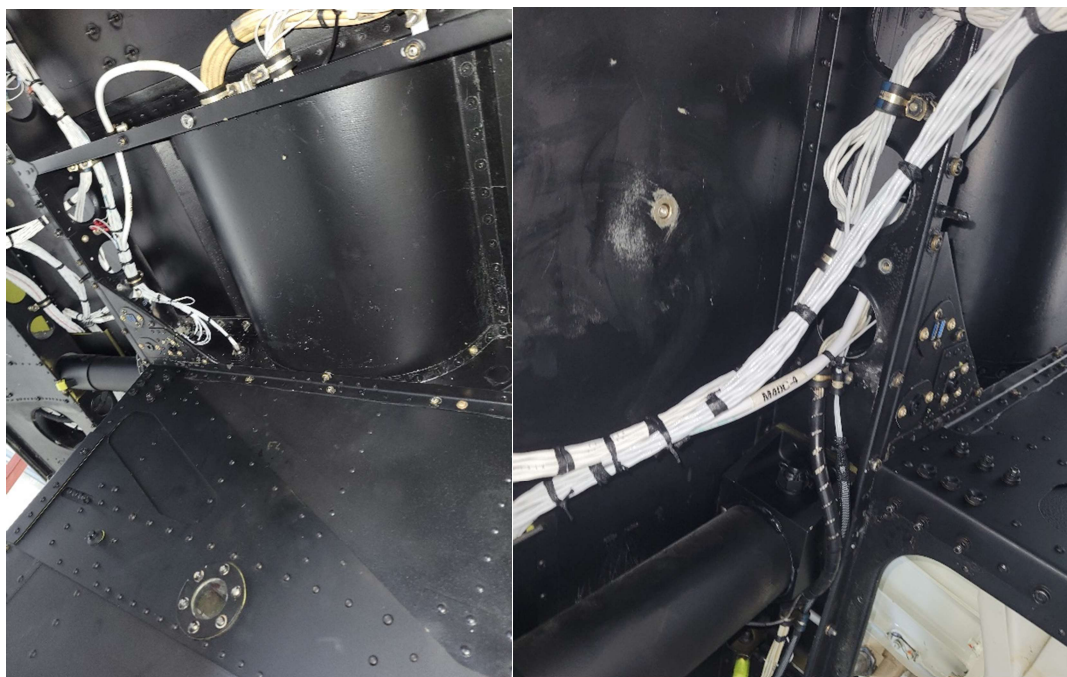
Figure 6.20: Ceiling routing from Hell Hole
